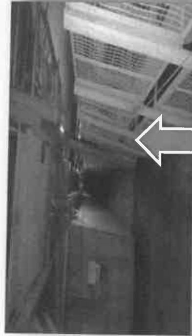
Closed conveyor belt in tunnel
