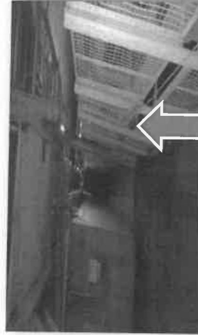
Under ground Tunnel provided to control dust emission
